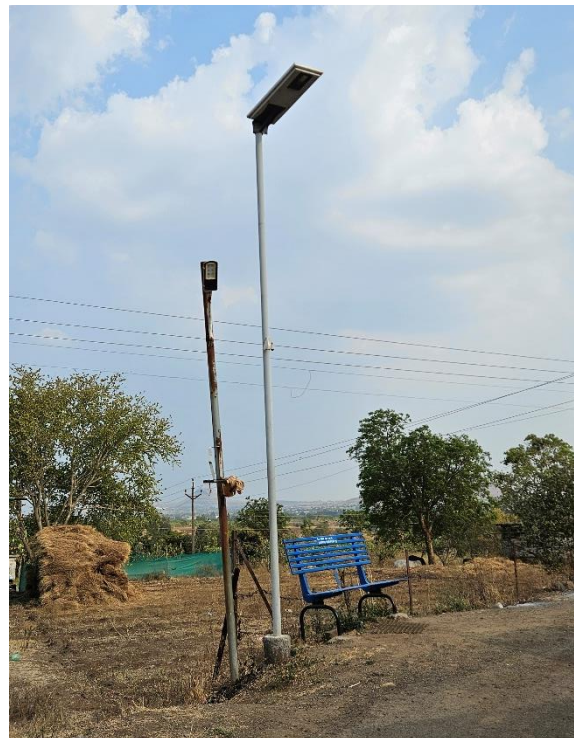
Figure 19: Solar streetlights installed in Madkijamb village
